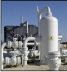
Wellsite initial separation
